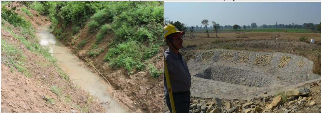
Garland DrainSettling Pond
