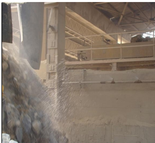
Water spraying System in Crusher Hopper
